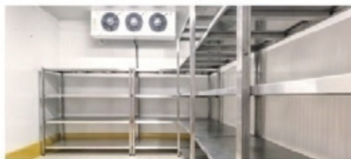
Restaurant cold rooms
